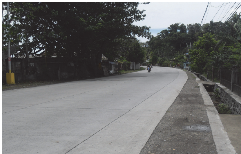
Figure 1-1: Jointed unreinforced concrete road with a tied concrete shoulder Design Standard DC7, Traffic Class T8
